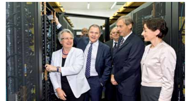
Figure 8: Ministers Schavan and Heubisch putting their hands on the warm-water cooling of SuperMUC.
